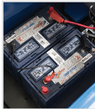
Battery Compartment The SA40™ is available with wet or AGM maintenance-free batteries.
