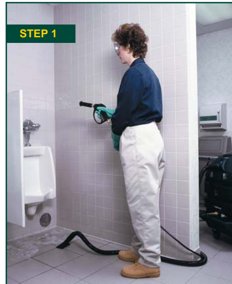
STEP 1 Use the low pressure trigger setting to apply Formula 710 Multi-Surface Acid Cleaner.
